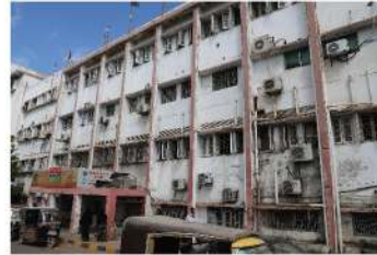
Upgradation and renovation of clinical laboratory/waiting area, CSSD and laundry at ground floor in progress.
