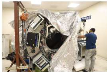
Installation of Second and more advanced unit of Tomotherapy in progress.
